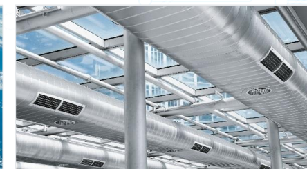
HVAC and Refrigeration
